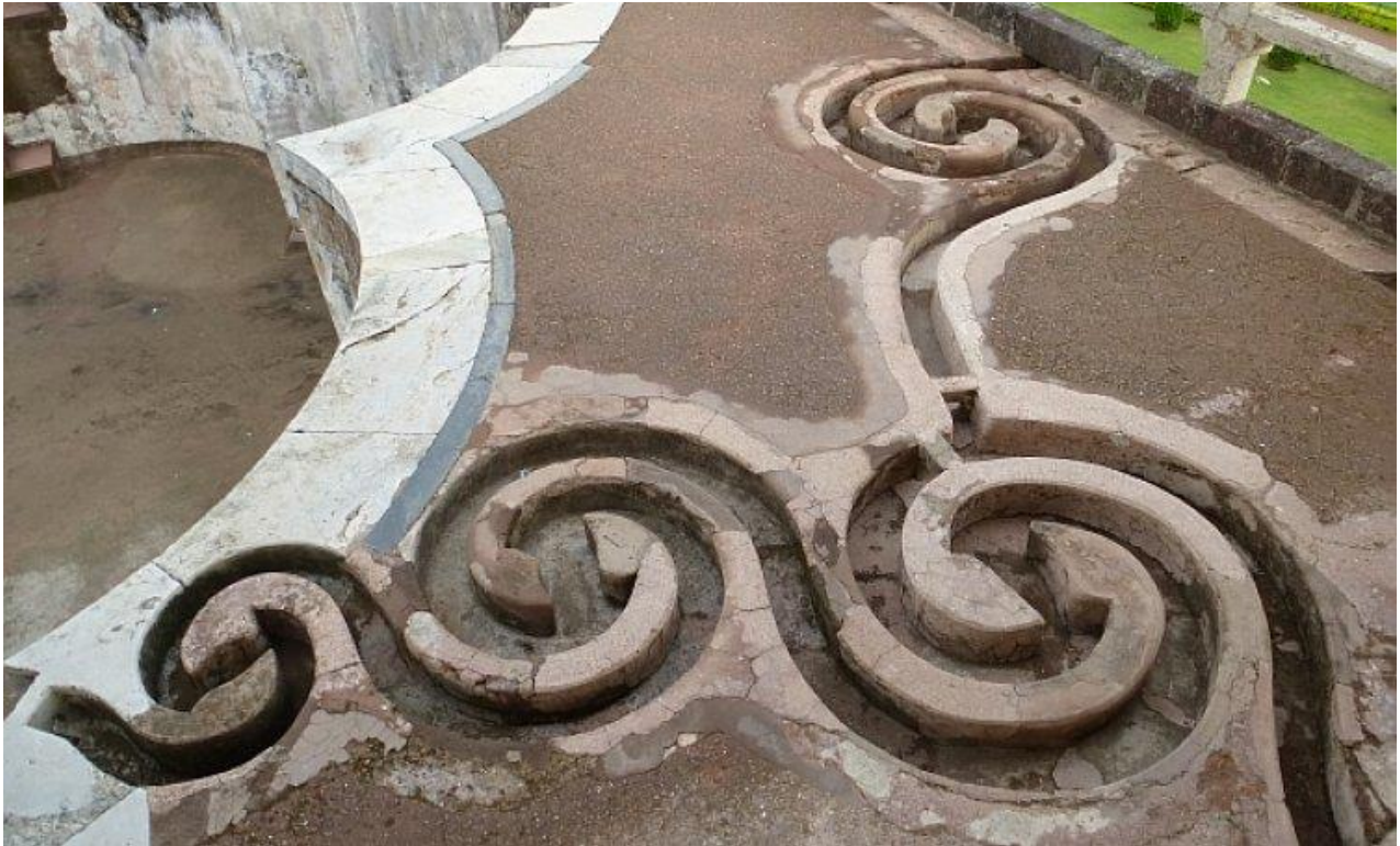
An intricate set of curlicues set in the floor leads rainwater from the roofs to a tank in Jahaz Mahal - Mandu Fort
